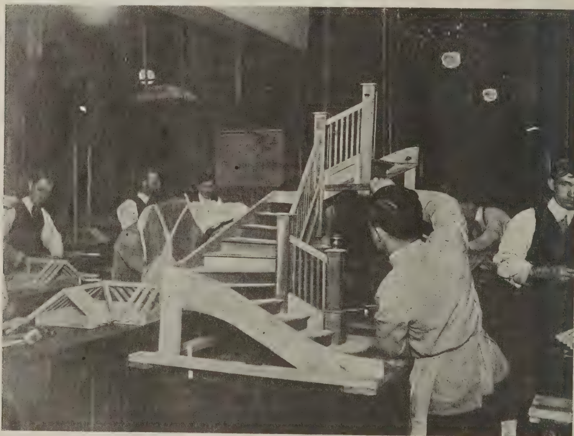
Fig. 31. The completed stair, one-third full size. A practical problem exemplifying many of the fundamental principles involved in the art of stair building
